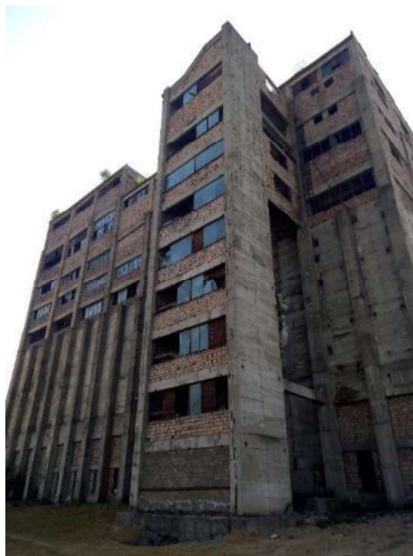
Figure 11. Overview of the sorting station [2]
