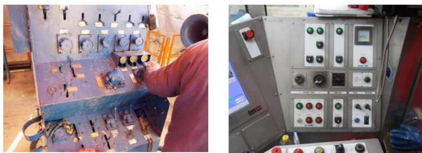
Figure 7. Control panels of used equipment
